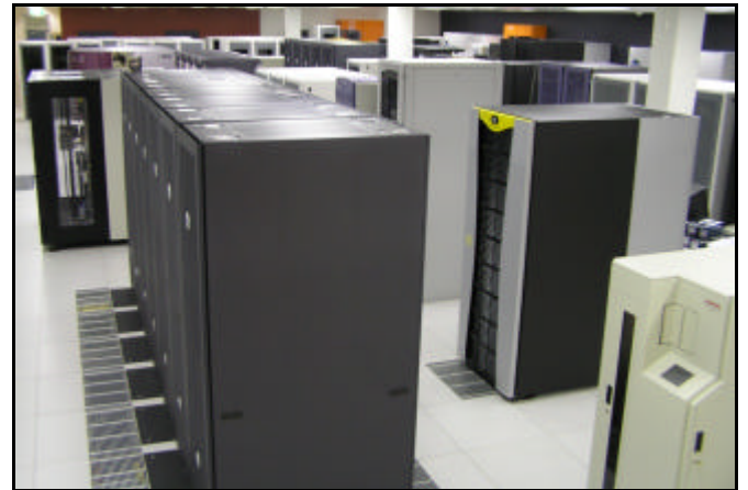
ac3 data centre at the Australian Technology Park
